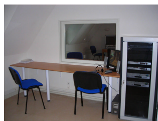
Technical room Saint Malo
